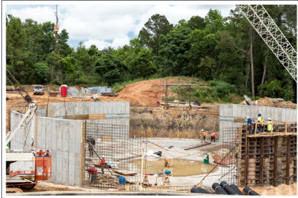
Omussee Creek WWTP under construction. Barge completed process and hydraulic modeling required to size treatment process components for this plant.
