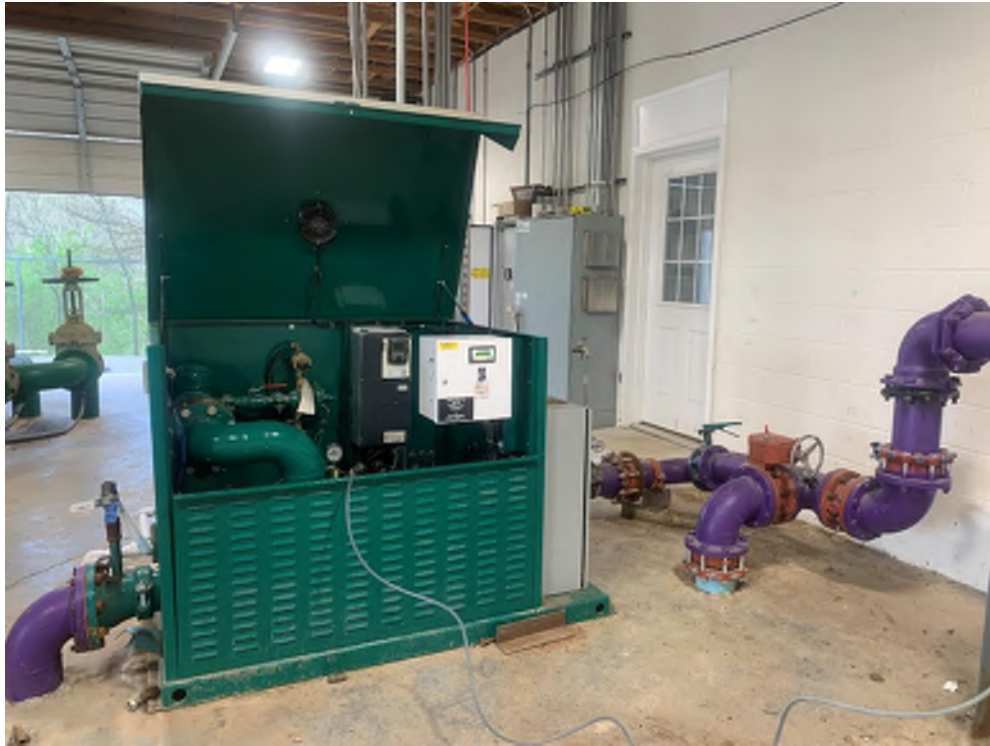
Figure 3.4 - Filtered Water Skid-Mounted Pump Station
