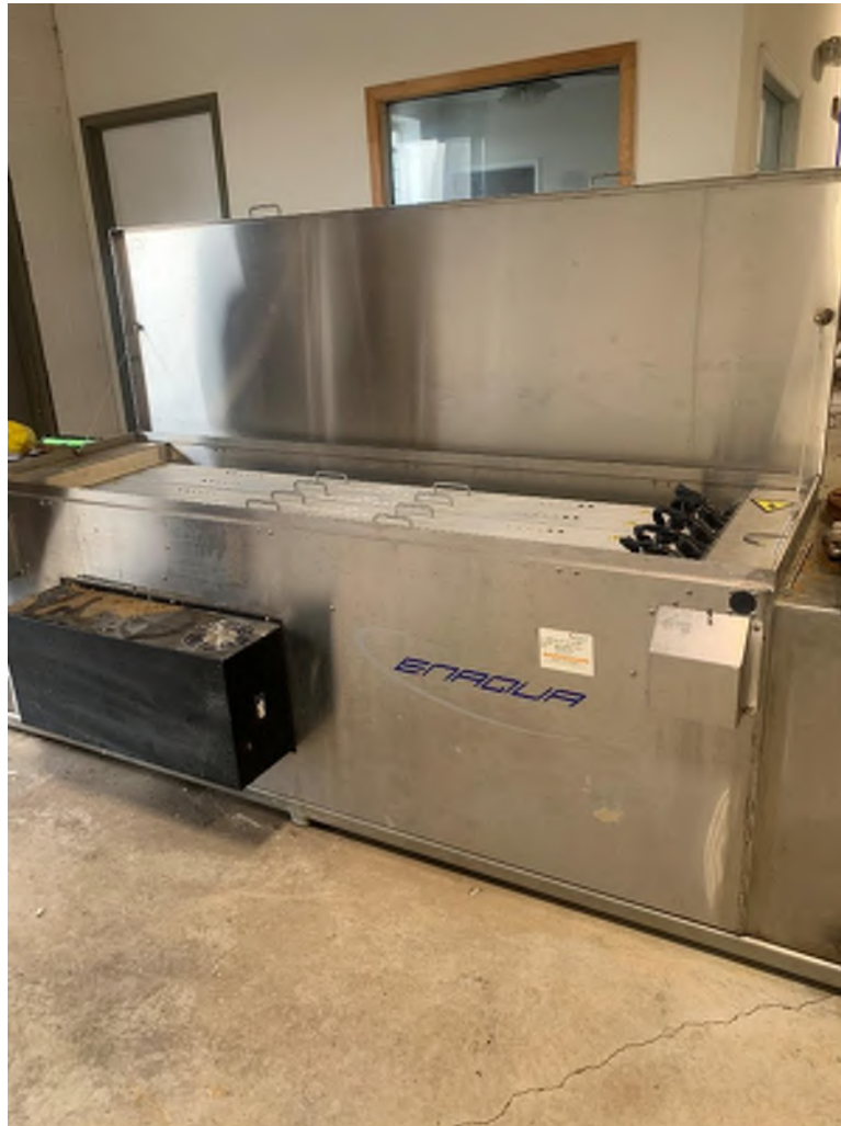
Figure 3.3 - Existing Ultraviolet Disinfection Unit
